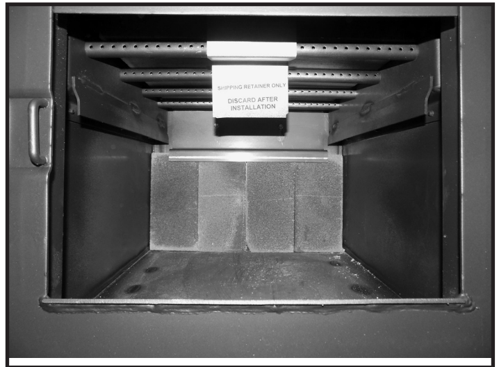
Figure 12: Bricks against rear wall.jpg
